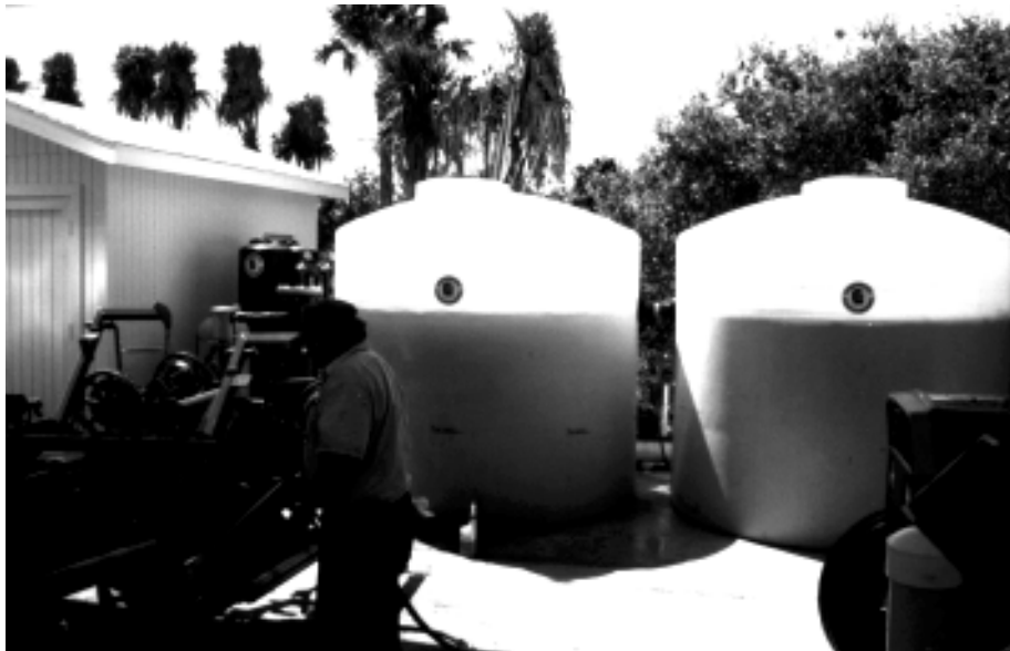
Figure 10. Wash water recycling system. Courtesy of Collier's Reserve.
